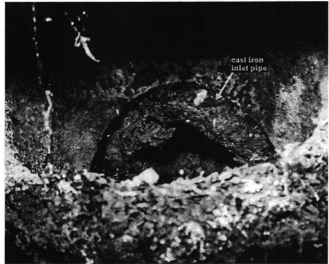
Septic System has a Metal Inlet Pipe.
