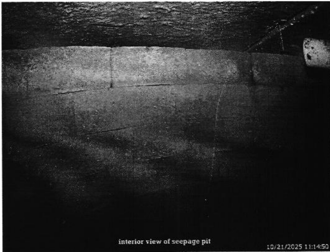
The seepage pit appears to be intact and functioning as intended at the time of the inspection.
