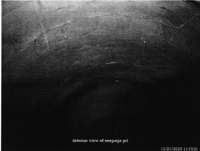
The seepage pit appears to be intact and functioning as intended at the time of the inspection.
