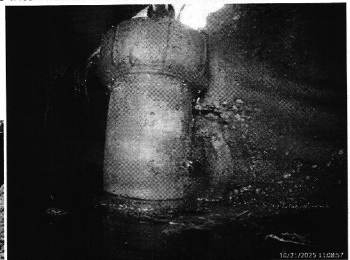
Outlet Baffle appears to be intact and working as intended at the time of the evaluation.
