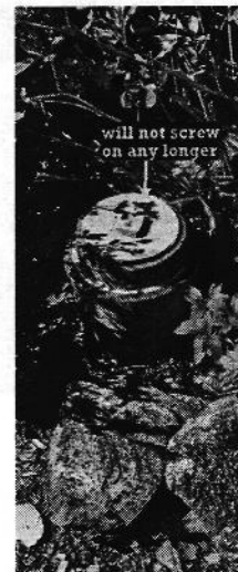
The cast iron inlet inspection pipe appears to be intact at the time of the inspection. However, the metal cap appears to be unable to screw into the top of the pipe and can easily fall or blow off and allow outside water or debris to enter the tank. Recommend a further evaluation from a licensed septic contractor to replace the cast iron inspection pipe.
