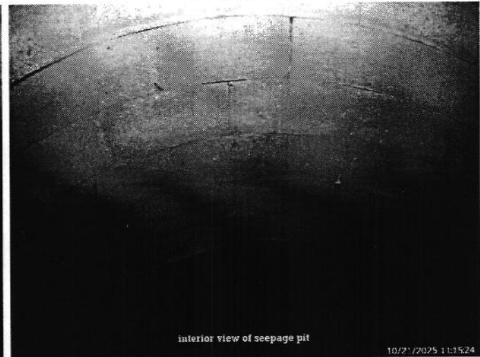
The seepage pit appears to be intact and functioning as intended at the time of the inspection.
