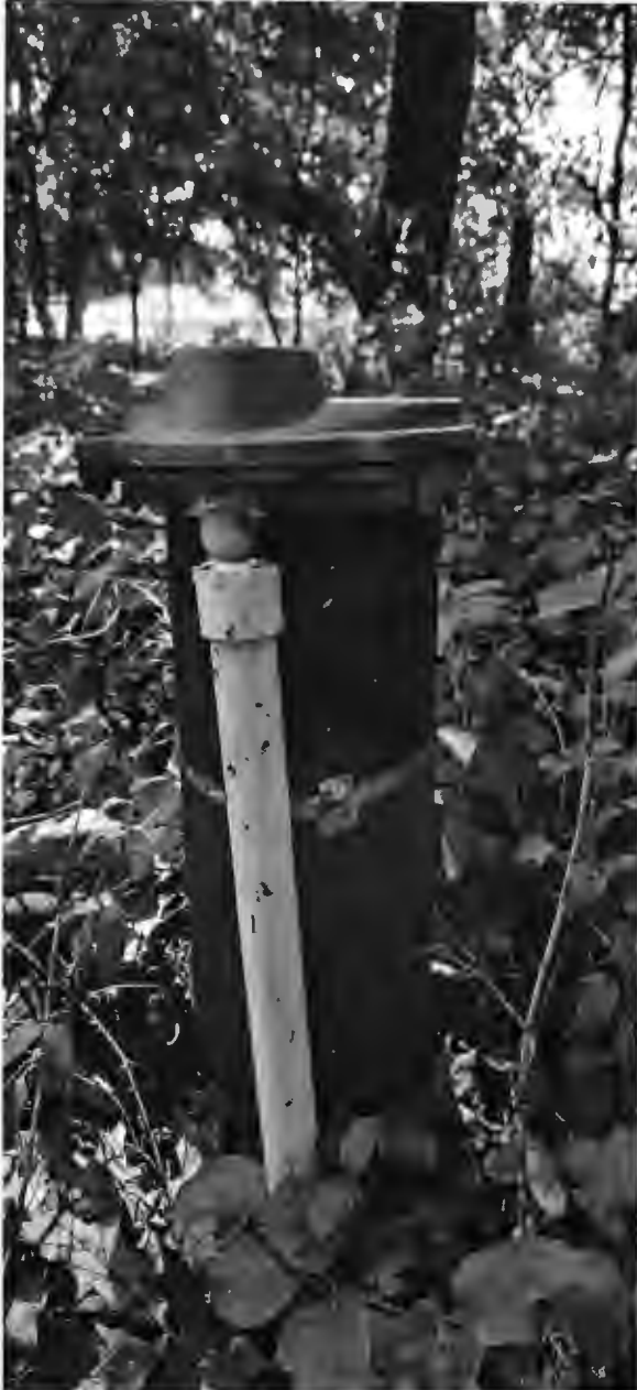
Well with broken conduit, missing bolt in cap and seal hanging out.
