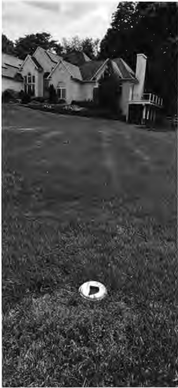
Septic tank clean-out with broken lid.
