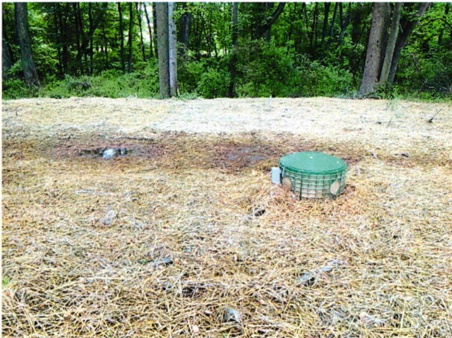
Ponding at upper edge of bed
