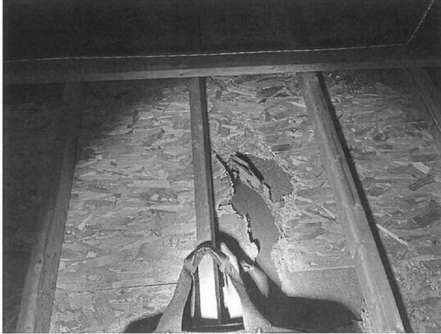
Photograph 9 - Damaged portion of OSB wall sheathing at right-side gable end wall of residence roof.
