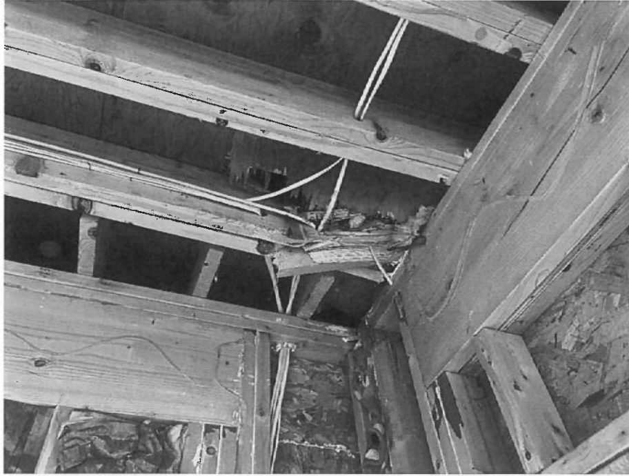
Photograph 5 - Damaged 2-ply 2x8 roof rafter and plywood roof sheathing for sunroom.
