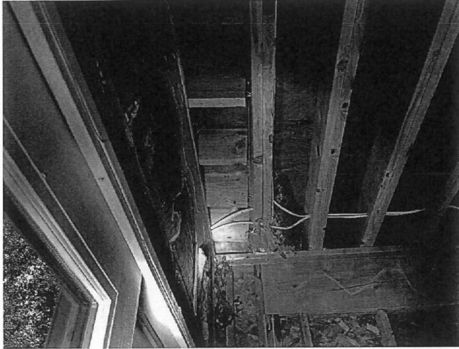
Photograph 7 - Detached 2x8 outriggers adjacent to damaged 2-ply 2x8 roof rafter.
