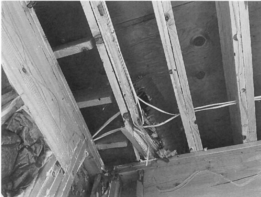
Photograph 6 - Damaged 2-ply 2x8 roof rafter and plywood roof sheathing for sunroom.
