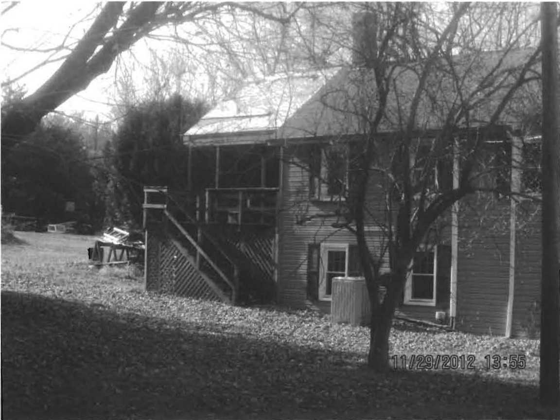
Roof system over deck built without permits or inspections. Roof system still in place 11-29-2012.
