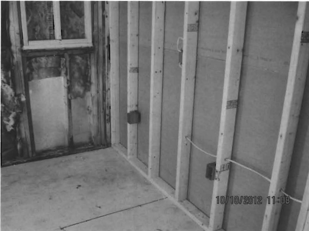
Interior alteration, kitchen location with new wiring; new plumbing will be required.
