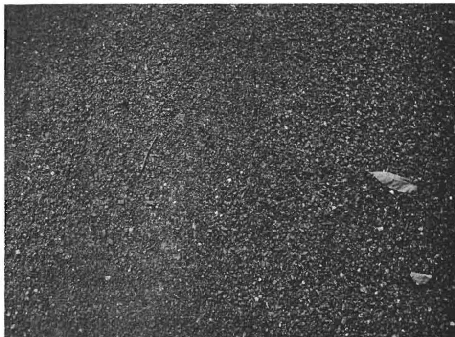
Tar and Chip Surface Treatment for Remainder of the Use-In-Common Driveway (Labeled as "Ex. Unpaved Driveway" on Exhibit B, except where indicated)
