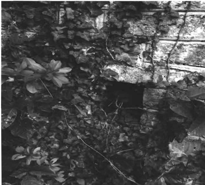
Photograph 7 Vent pipe for the heating oil UST in the wall of the residence
