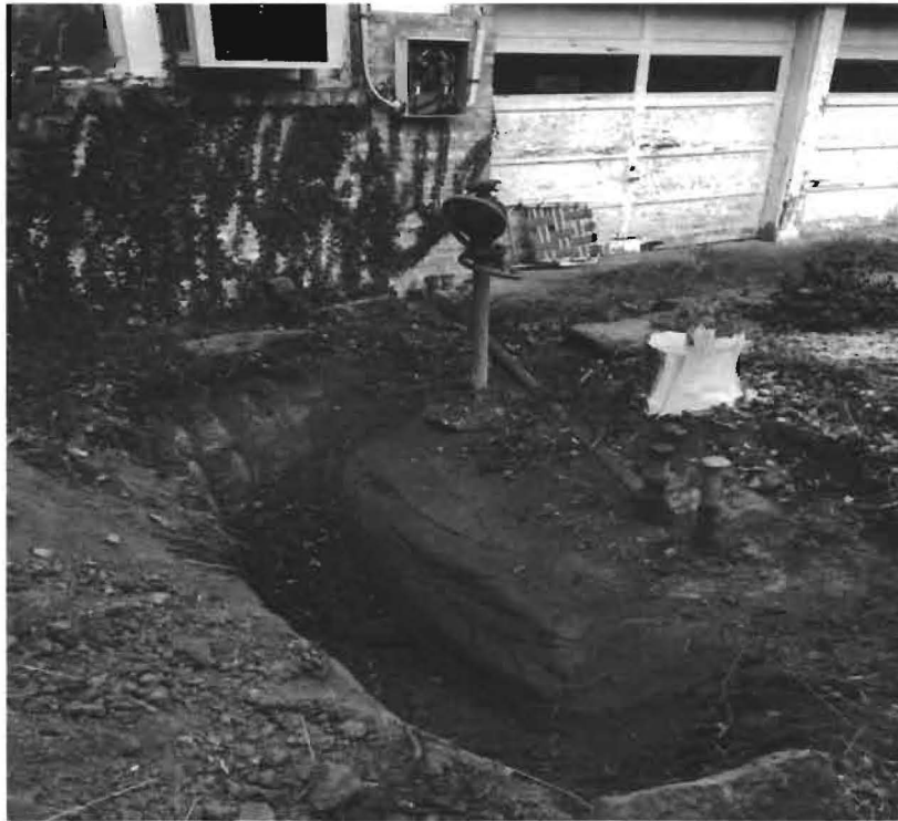
Photograph 1 Diesel UST located on the northwestern side of the residence
