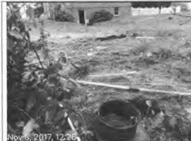
Picture 2: The drywell is approximately 6 feet off the back of the septic tank.
