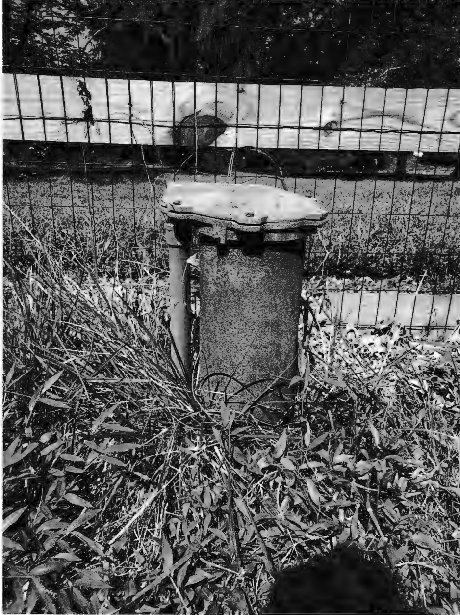
Existing well. No tag. Two-piece cap and electrical conduit secured. No noted issues.
