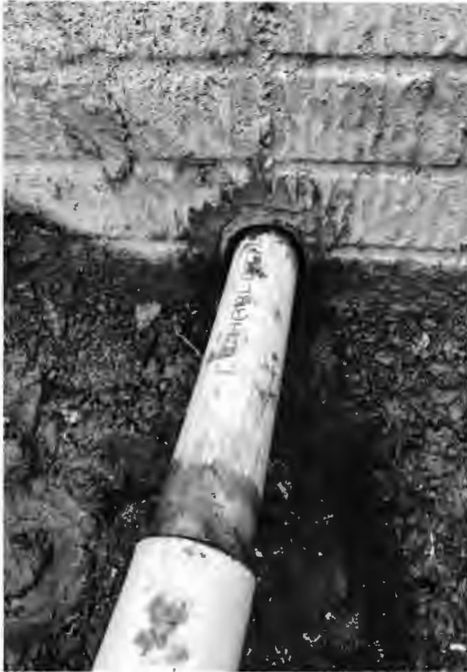
Builder has base sealed inside the house. Builder will also seal outside. (18)
