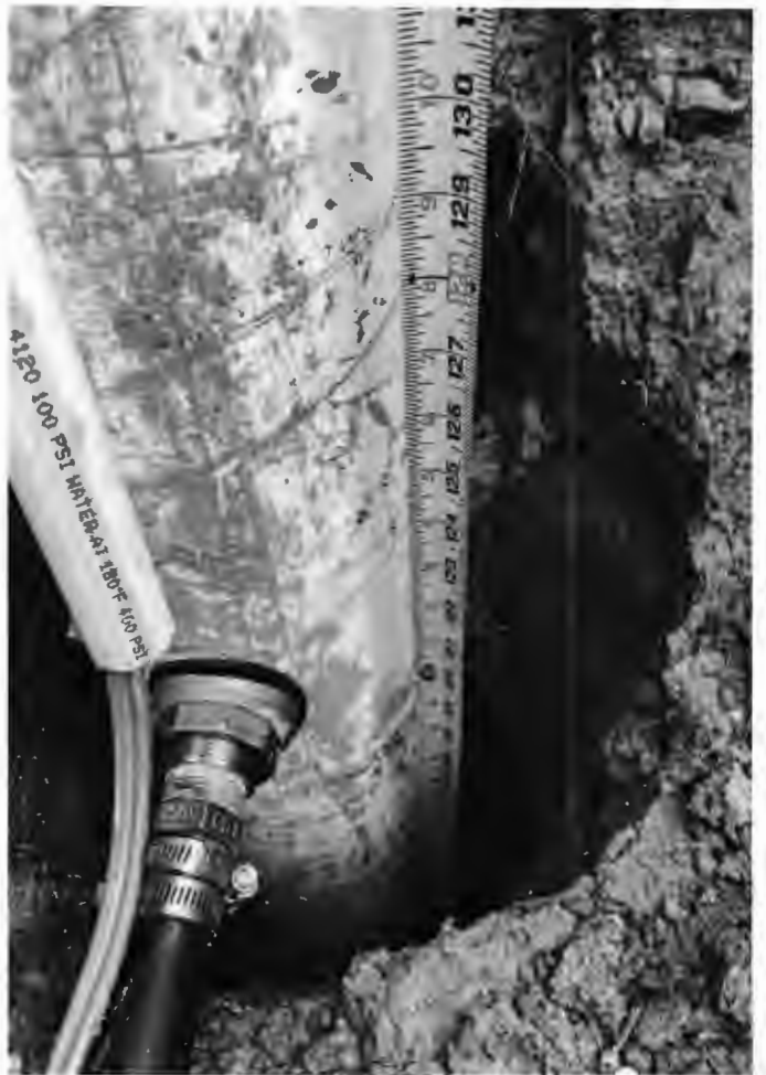
Grout has settled 10' below process adaptor. Well drilled to seal grout void. (18)
