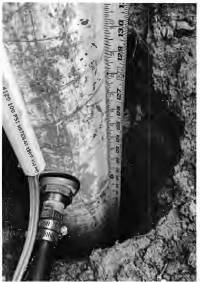
Grout has settled 10' below process adaptor. Well drilled to soil grout void. (18)
