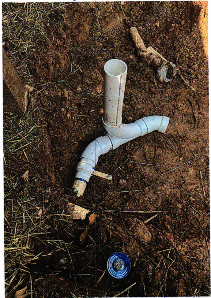
Front line originally was 3". Contractor ferroced to 4". (MB)
