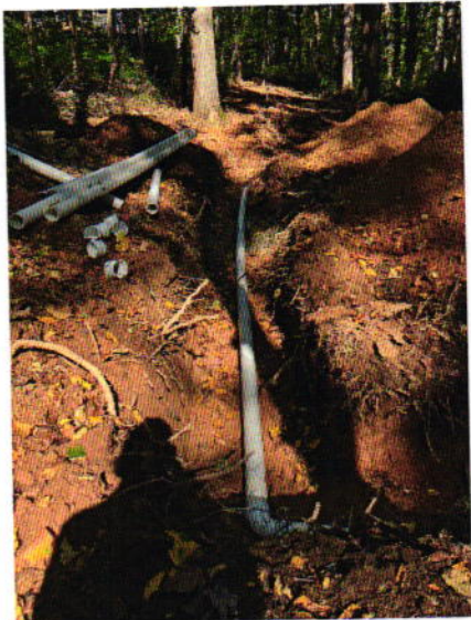
Rock @ 4" outlet line
