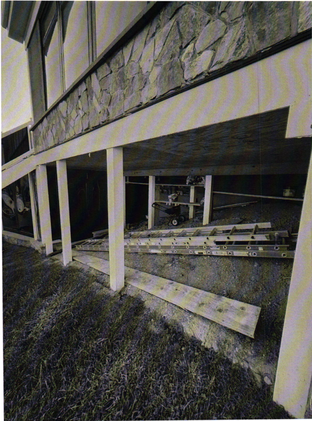
Structural support of Sunroom and void under – void not converted.
