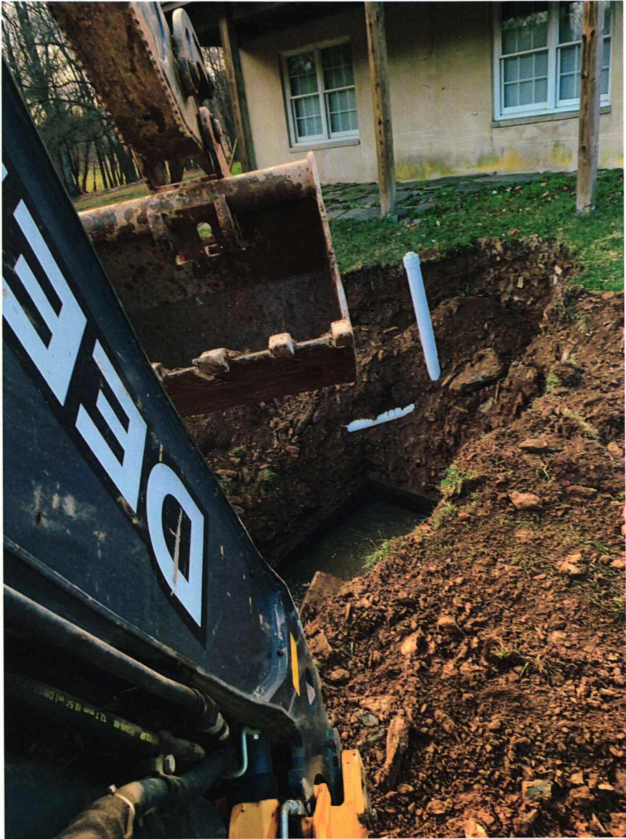
12/17/2025 - picture of tank From installer. (SP)
