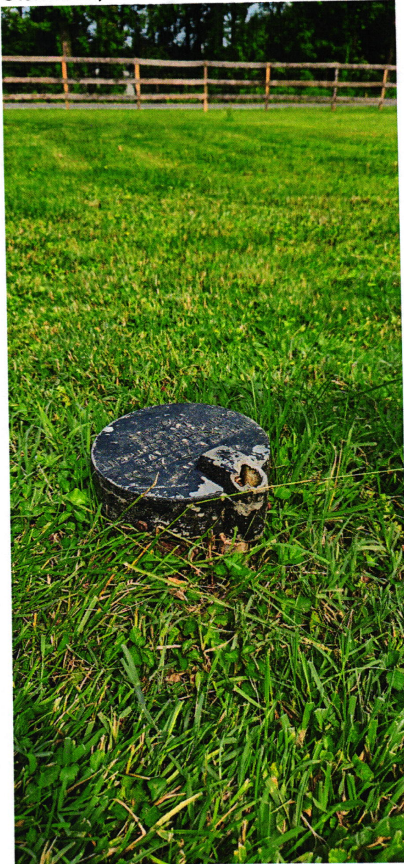
1 pc cap with hole in it. pvc conduit is not flush with cap.
