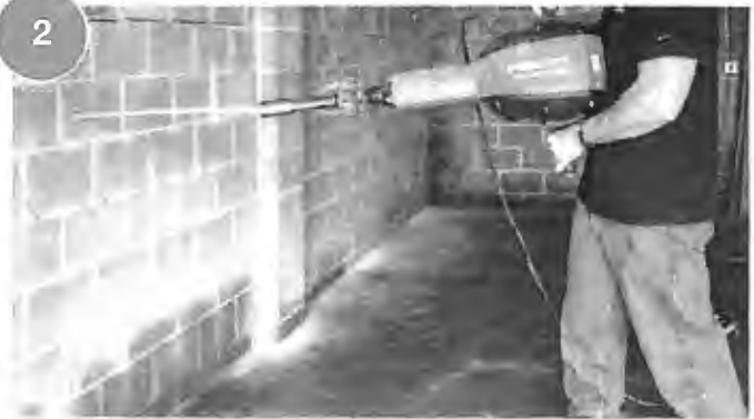
2 Drive galvanized steel rod through small hole in foundation wall and attach to earth anchor.
