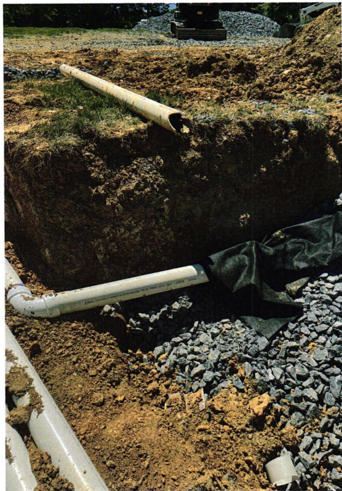
Upper trench does not have adequate stone, pipe is on side of trench
