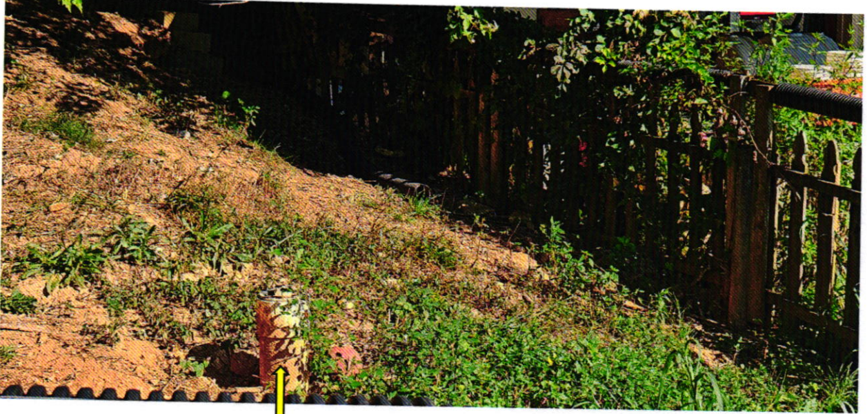
Drywell clean-out for house .
