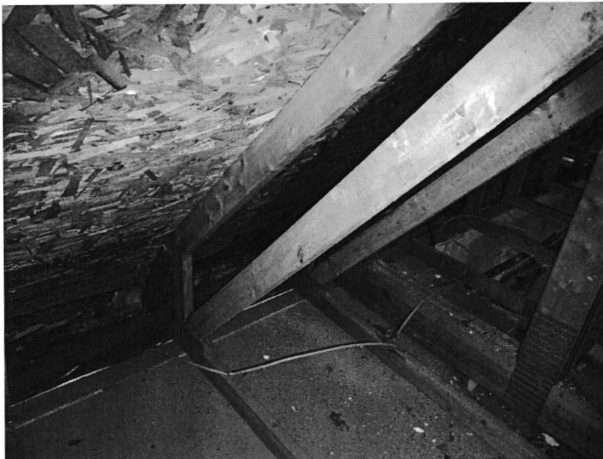
Photograph 8 - View of damaged roof truss.
