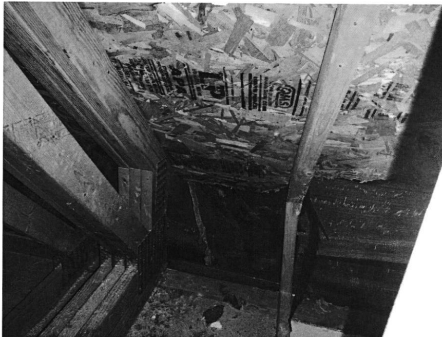
Photograph 6 - View of damaged jack truss.
