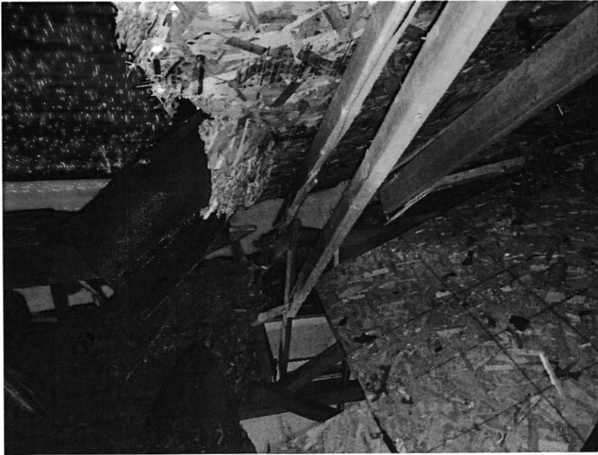
Photograph 11 - View of damaged roof sheathing and displaced roof rafter
