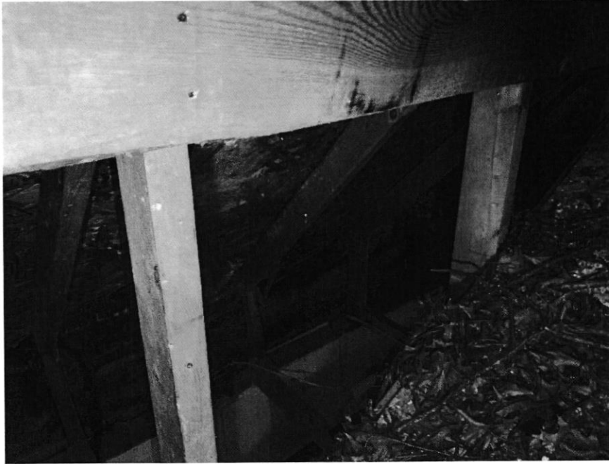
Photograph 7 - View of damaged jack trusses.
