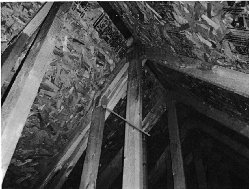
Photograph 12 - View of displaced metal plate on front overbuild truss.
