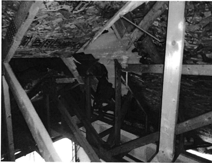
Photograph 5 - View of damaged 2-ply girder truss and stepdown truss on the left-hand side of the garage.
