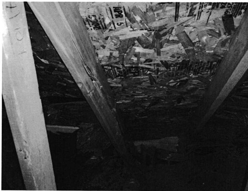
Photograph 9 - View of damaged roof rafters and OSB sheathing.
