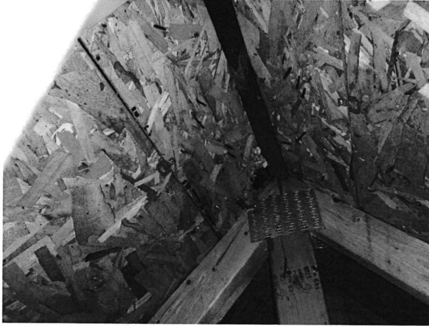
Photograph 13 - View of branch puncture.
