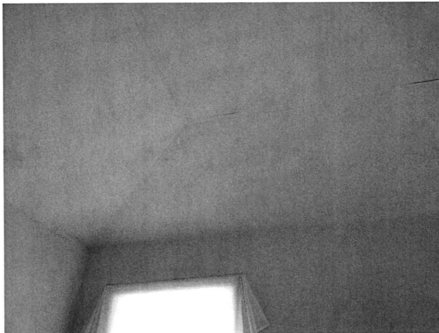
Photograph 16 - View of damaged drywall seam in left-rear bedroom.
