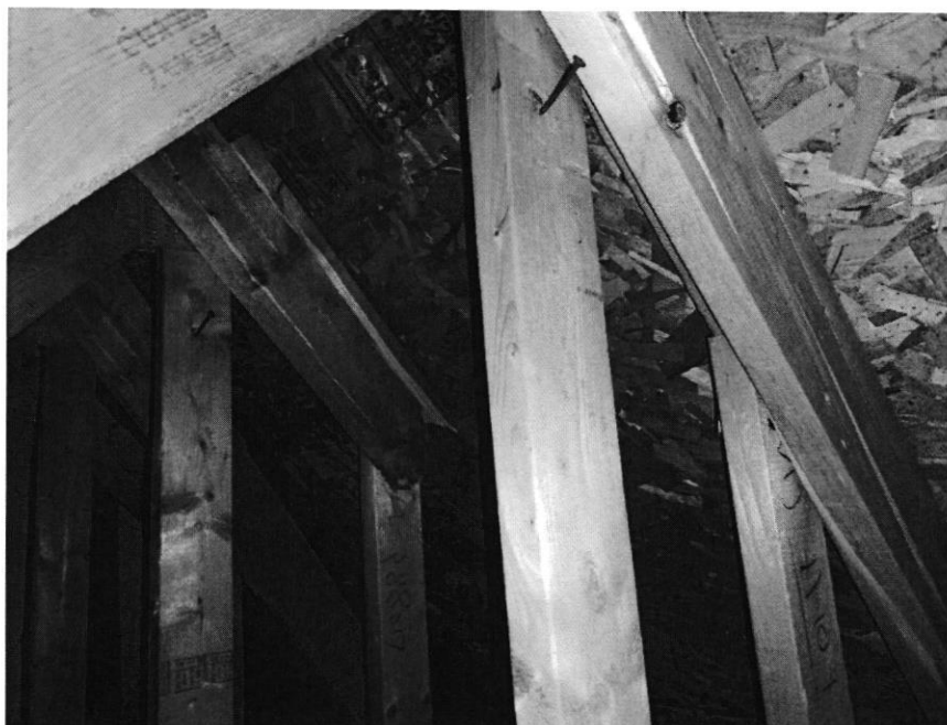
Photograph 10 - View of fractured 2x6 roof rafters.
